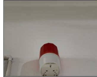
Photo of fire safety equipment 4.2_Fire_alarm.jpg
