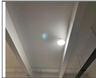
Photo of non-conformity 5.1_Ordinary_fluorescent_lighting_used_in_the_warehouse.jpg
