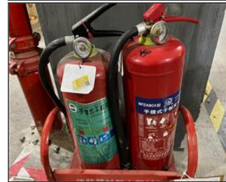
Photo of fire safety equipment 4.6_Fire_extinguishers.jpg
