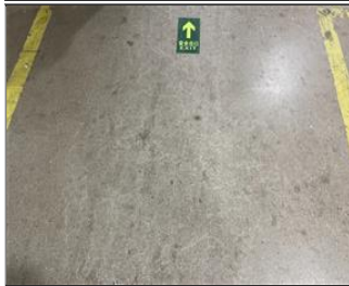
Photo of fire safety equipment 4.6_Exit_route_with_marking.jpg
