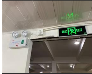
Photo of fire safety equipment 4.1_Exit_sign_and_emergency_light.jpg
