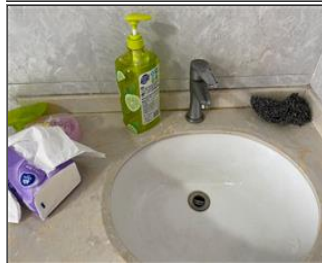
Photo of the sanitary facilities 13.2_Photo_of_the_sanitary_facilities.jpg
