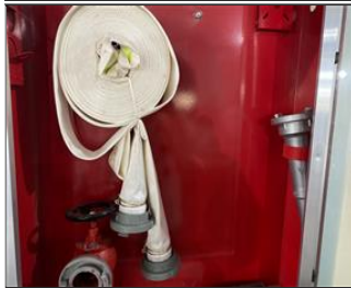
Photo of fire safety equipment 4.3_Fire_hydrant.jpg
